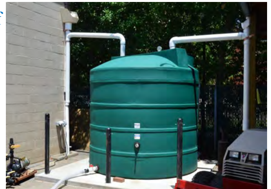
Cistern installed at UNC-G to collect rainwater.
