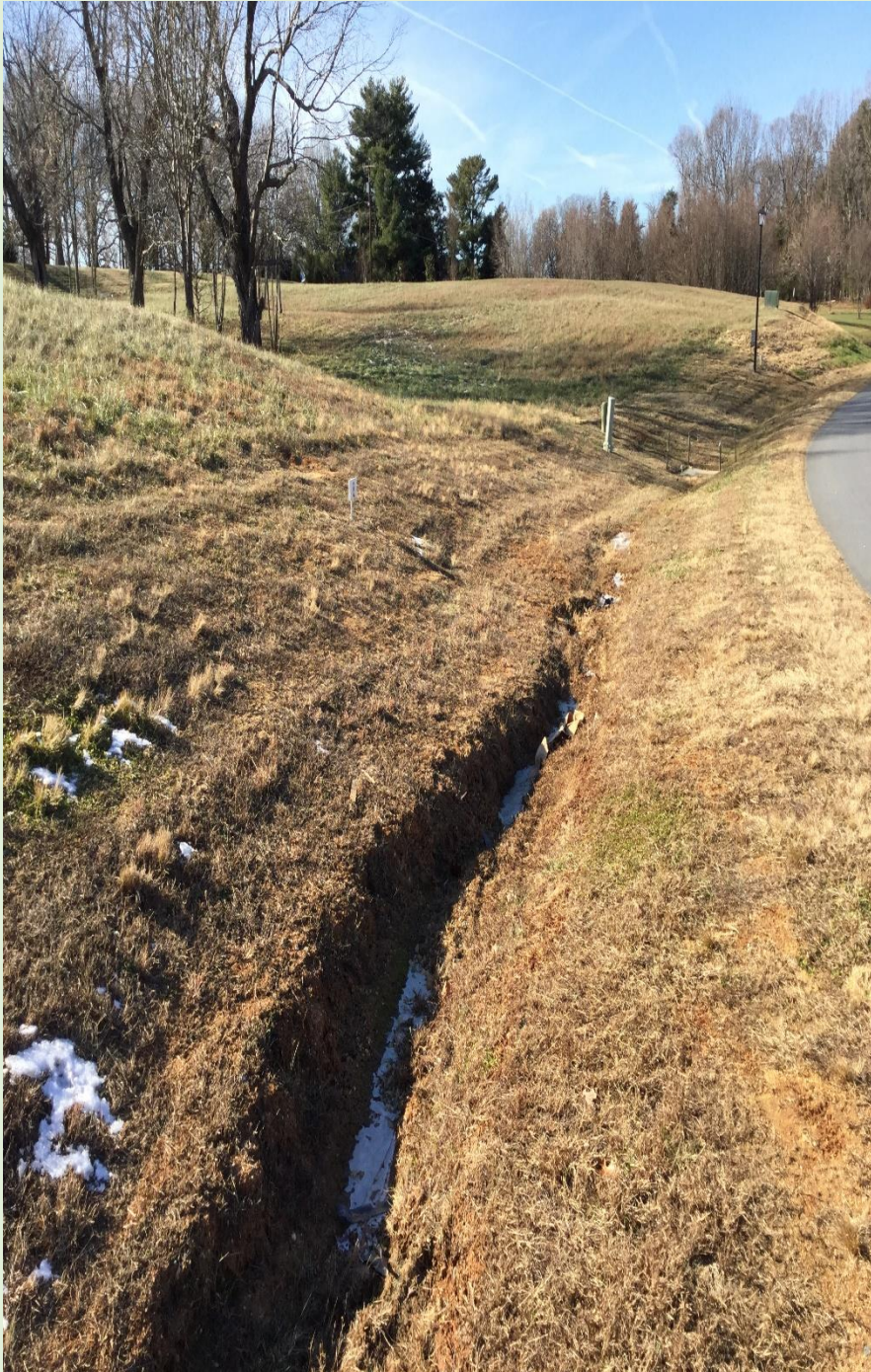
Bare and eroded side ditches of public streets.
