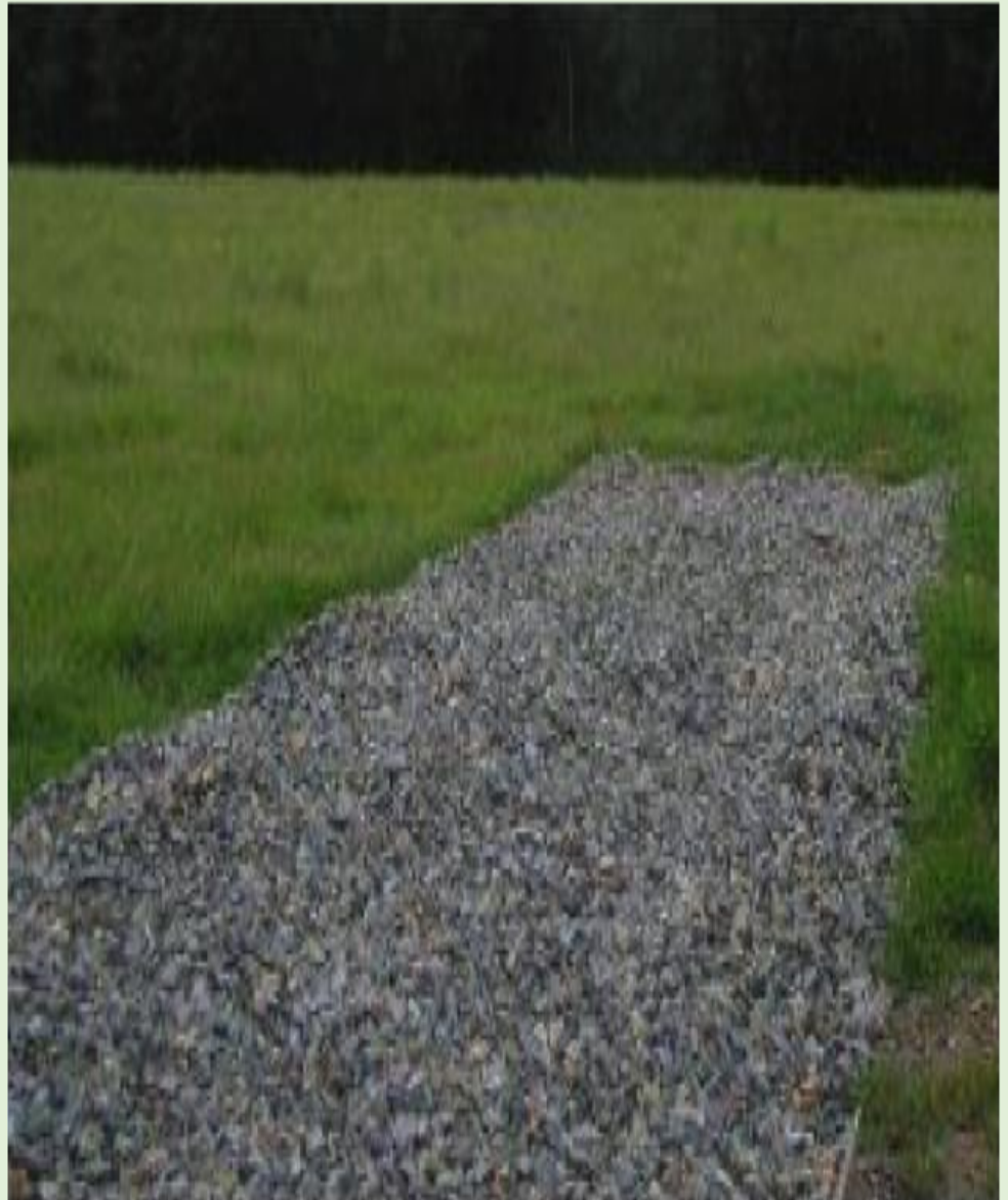
Install a temporary gravel construction entrance/ exit. This will provide a buffer area where vehicles can drop their mud and sediment to avoid transporting it onto public road, to control erosion from surface runoff, and to help control dust.
