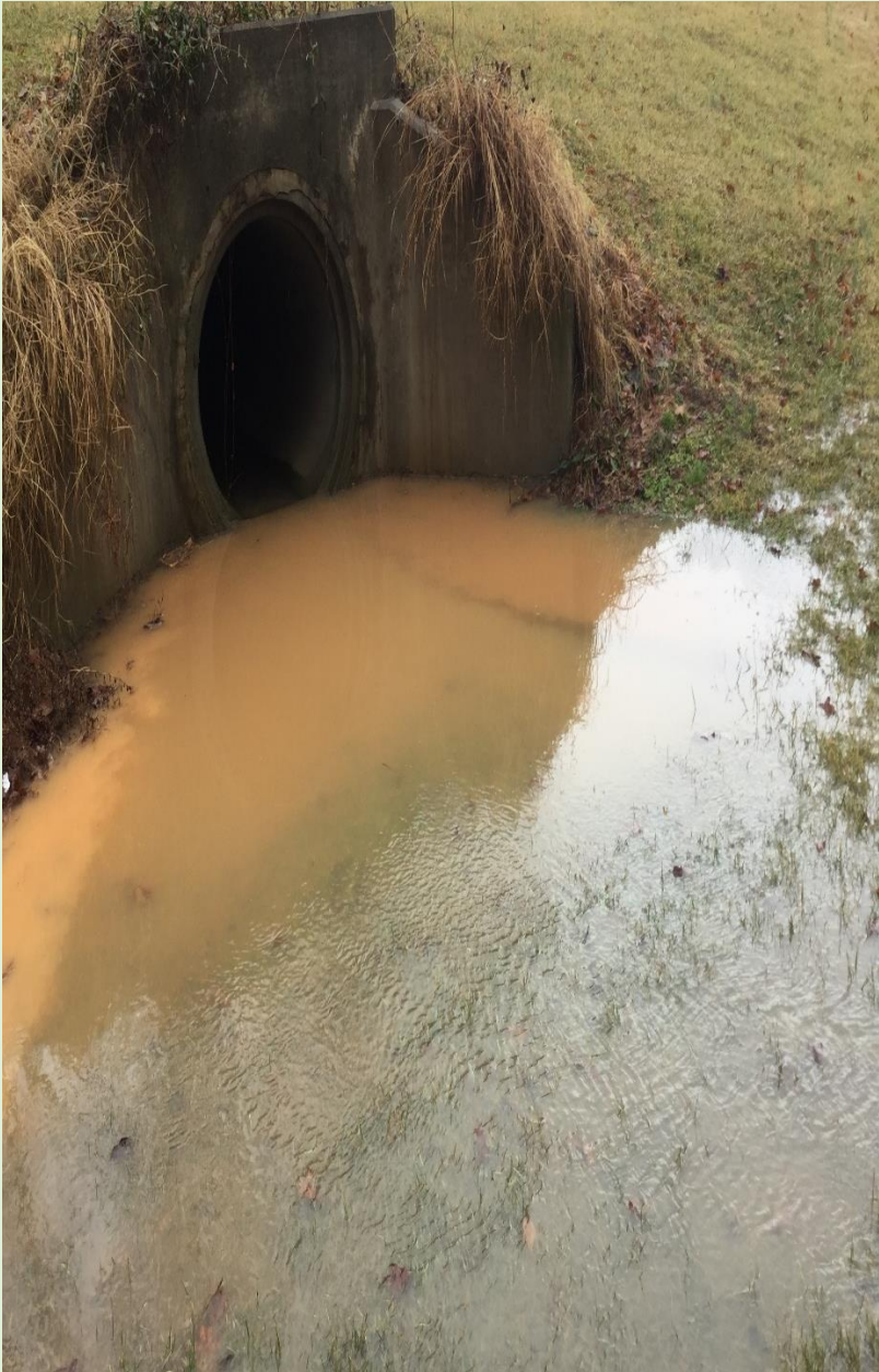
Mud and silt obstructing drainage culverts.
